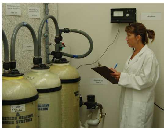
Large water purification system.
