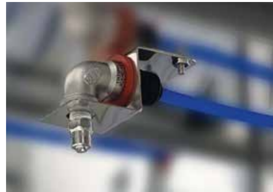
Programmable water spray periods can operate during either the light or dark periods.
