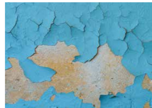
Water plays a role in many different physical and chemical failure modes.
